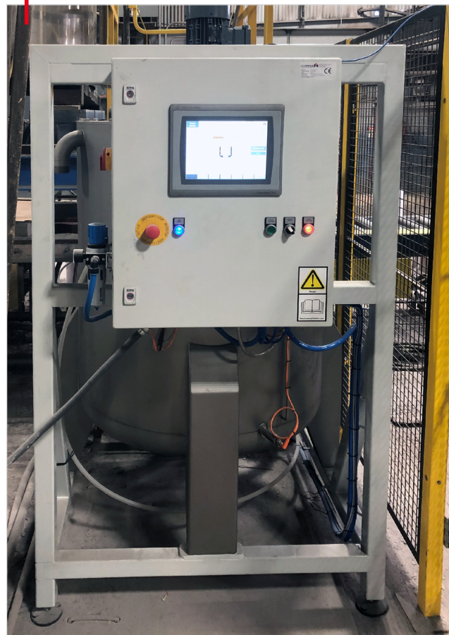
ICU-Modular unit located by spray line
